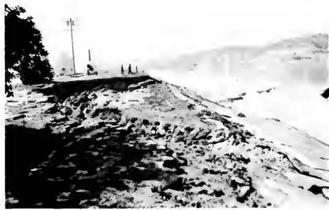
Photo 11. View south shows landslide in west side of small peninsula extending out into Upper Van Norman Reservoir; this area is part of fill at north edge of reservoir which failed (locality 13, plate 3). Photo by James E. Kahle.
